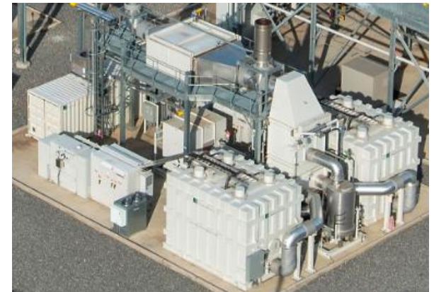
Carbonate Fuel Cell Powerplant
