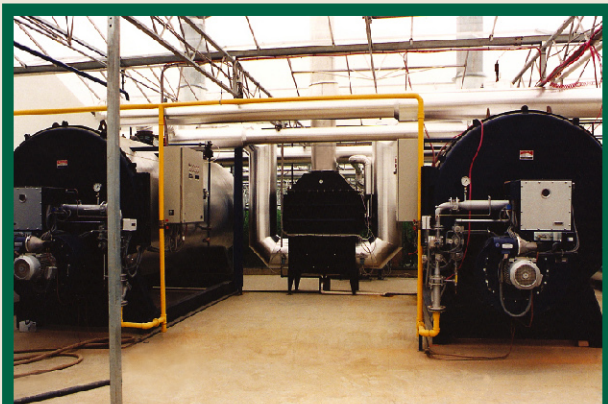
Waste Heat Recovery Unit
