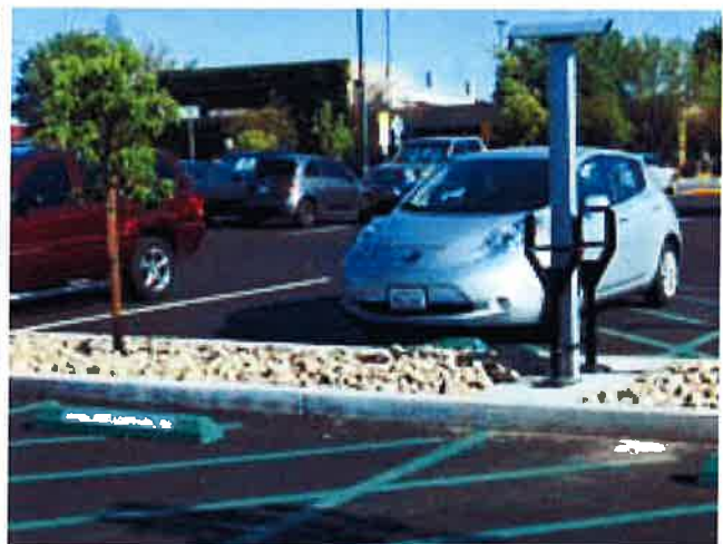
Electric charging station in Bakersfield
