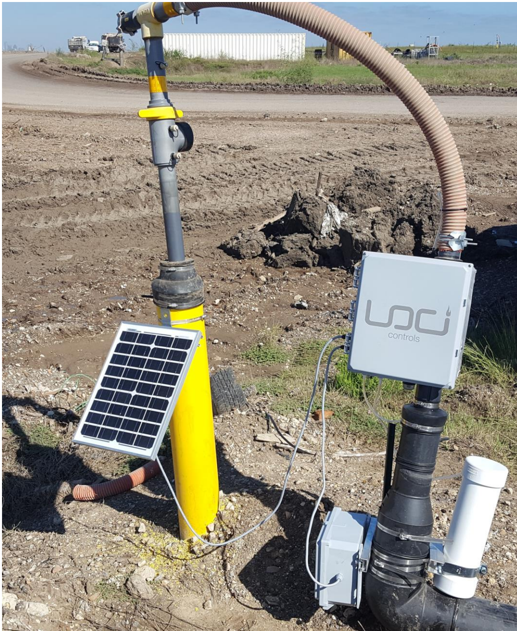
Photo 1: Loci Controller unit on well at the McCommas Bluff landfill in 2018
